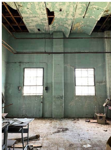
Photo 6: Building 12A interior, with collapsed ceiling, cracked ACM floor tile, peeling paint, and cracked concrete frame at windows.
