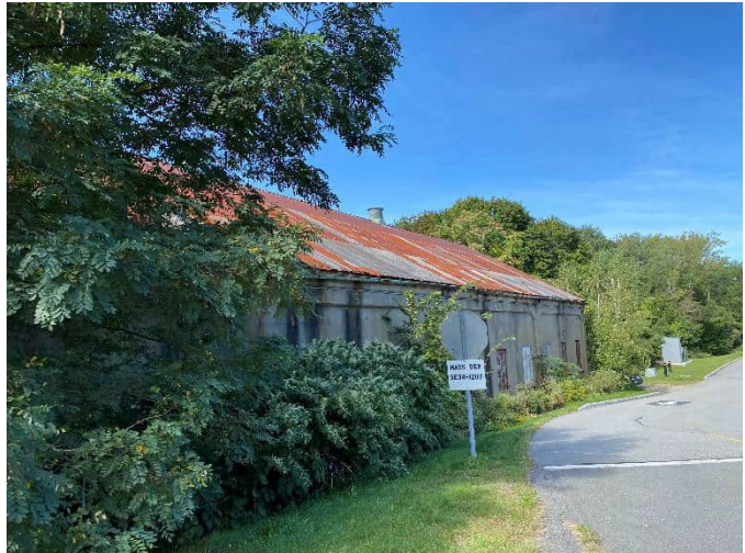
Photo 2: East elevation – note significant rust on corrugated metal roof.
