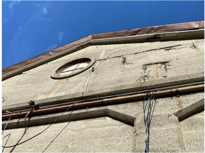
Photo 4: Concrete frame has numerous areas of spalled and cracked concrete, with rusted and exposed reinforcing.
