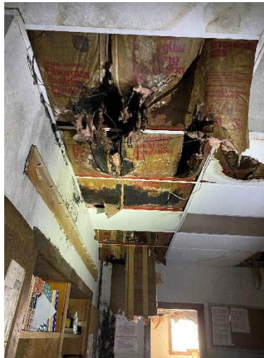
Photo 5: Ceiling of Building 12A in former wood shop, with numerous roof leaks, failed ceilings and moldy insulation.
