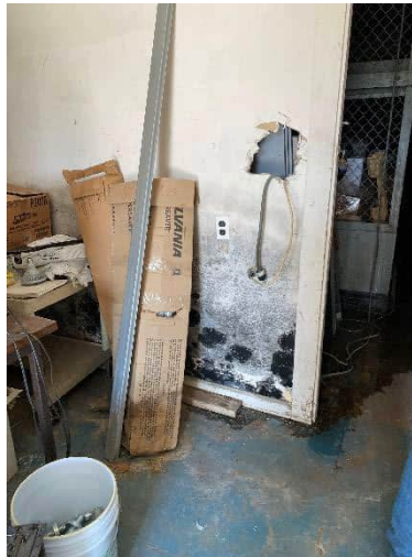
Photo 8: Extensive roof leaks and mold throughout Building 12B, which is filled with old desks, chairs, partitions and kitchen equipment.
